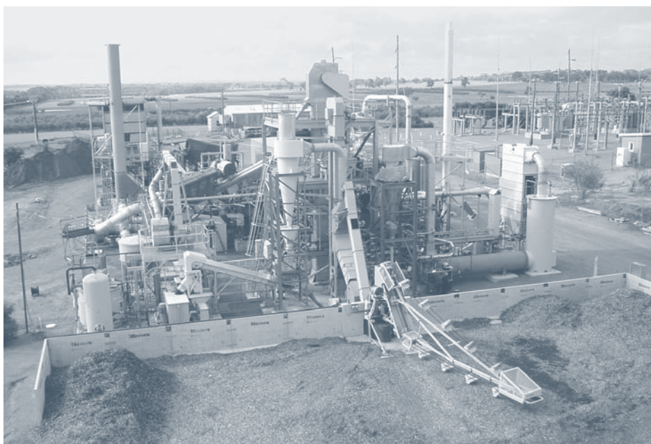
Aerial view of the integrated wood processing demonstration plant at Narrogin, Western Australia. Photo: Verve Energy
