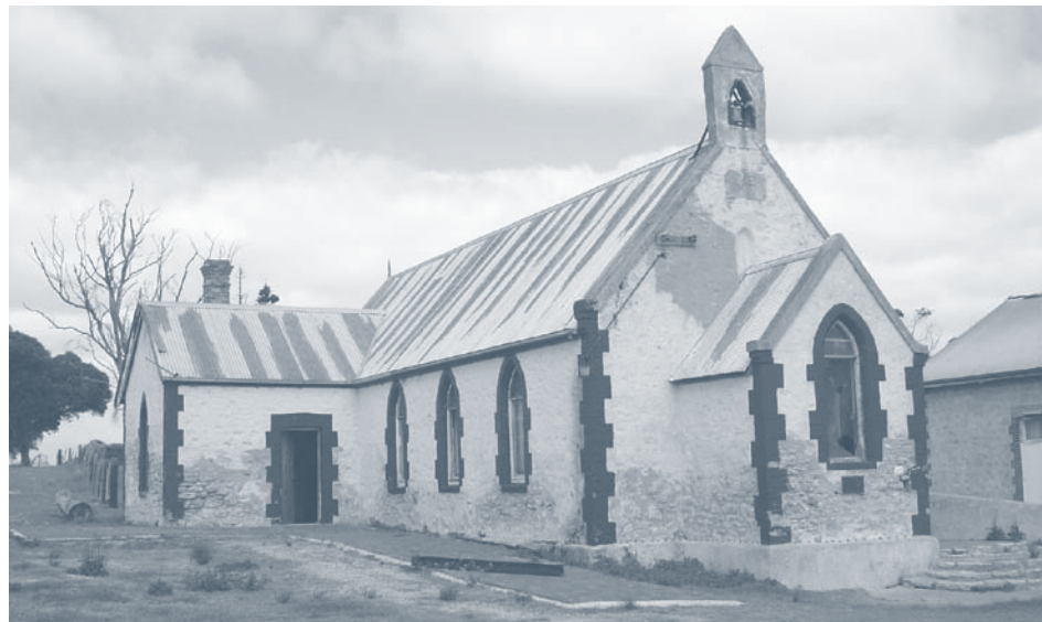
Restoration of the historic church at Raukkan (Port McLeay) in South Australia, which features on the Australian $50 note, is being funded by the Indigenous Heritage Programme through a Shared Responsibility Agreement with the Raukkan community. Photo: Brian Prince
