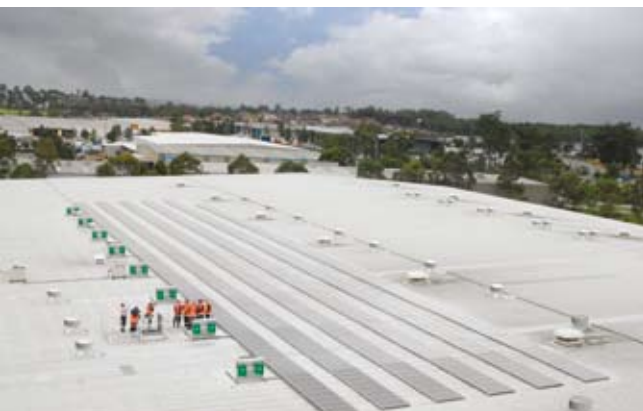
100Kw solar system on the roof of Cadbury Schweppes factory, Blacktown Solar City. Photo: Courtesy of BP Solar
