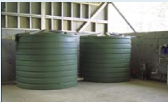
Stormwater holding tanks at new nursery.
