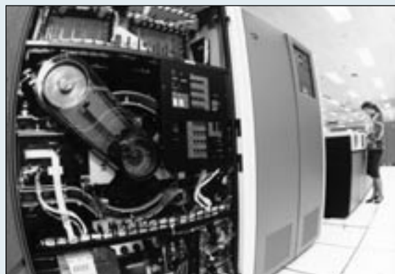
Communications Centre – Computer Room 2.
