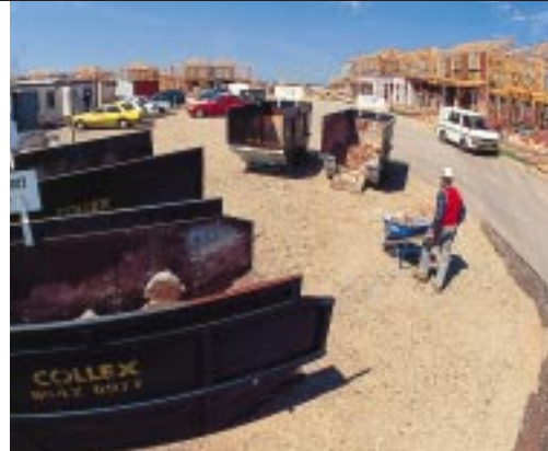
Partners in the WasteWise Construction Program manage waste at the Sydney Olympics Site.
