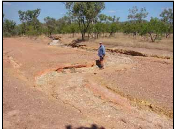
Image 2 – More washouts on the road to Maguk Further roadworks will be required to repair this washout.
