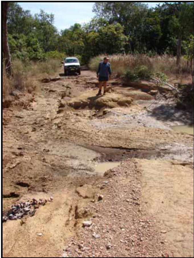
Image 1 – Washouts on the road to Maguk Roadworks are required to repair two sites along this track.
