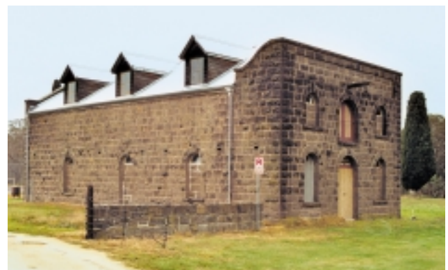
Cobb & Co. Changing Station, Buangor, Vic. This coach and livery station dates from the 1860s. It has been modified for other uses but is now vacant.
