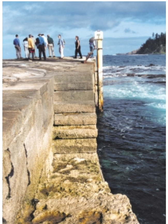
The Norfolk Island convict-built pier being inspected for urgent repairs. It has been in constant use for more than 150 years.
