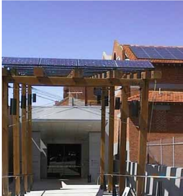
Figure 5: Moreland City Council Solar Pergola
