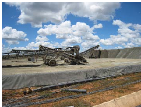
Figure 5.3 Stockpiling of ore on the heap leach pad at Caetite uranium mine, Bahia, Brazil
