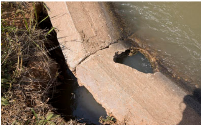
Damaged irrigation channel (M Mohell)
