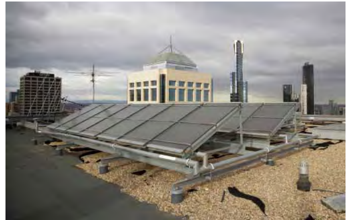
Photovoltaic rooftop solar panels in a busy city hub (Lauthier & DEWHA)
