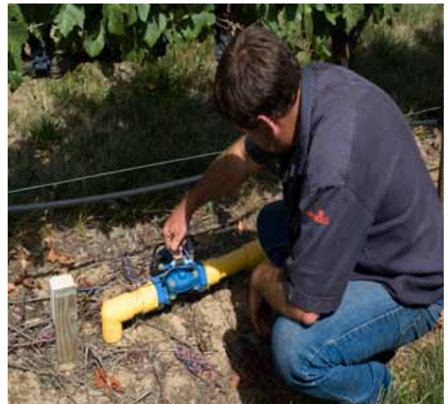
Irrigation regulating valve for further refining volume of water (J Baker)
